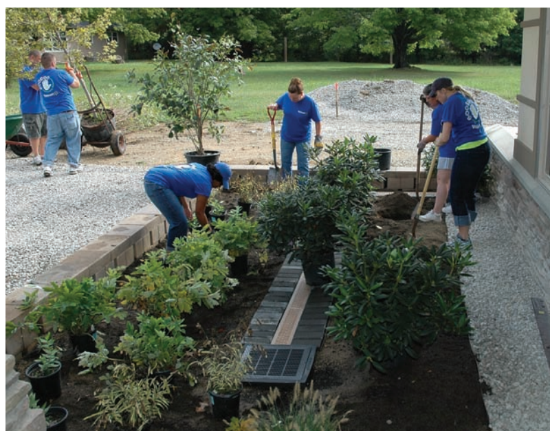
Above: Walmart employees volunteered to plant the trees and shrubs. This front landscape bed was filled with a premium soil mix prior to planting. Top: This captured rainwater will irrigate the landscape. The 20-foot stream assists in aerating and filtering the stored rainwater, while providing beauty and soothing sounds.
