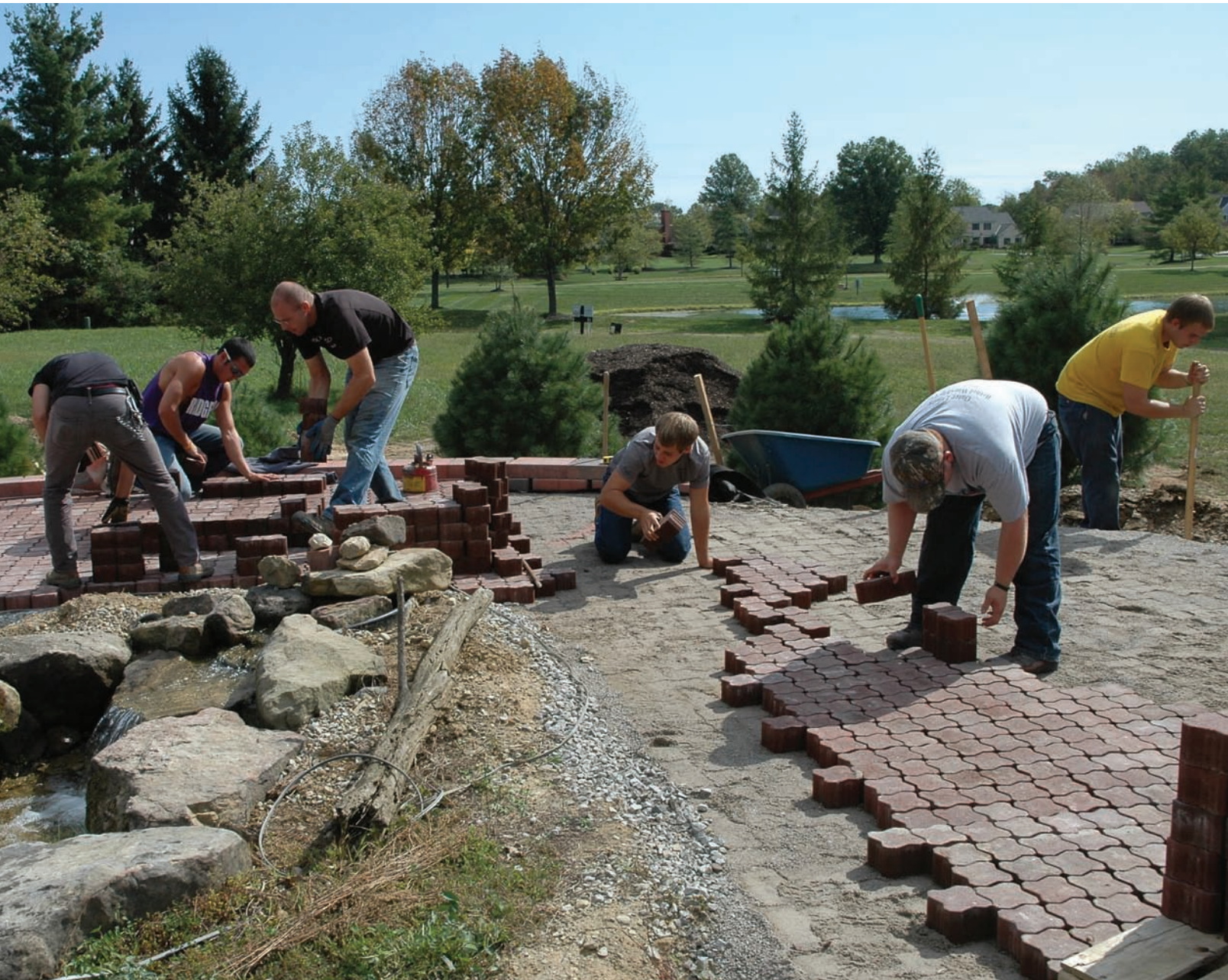
Hocking College students installed pavers on the upper deck. Students worked at the Universal Design Living Laboratory on several occasions.
